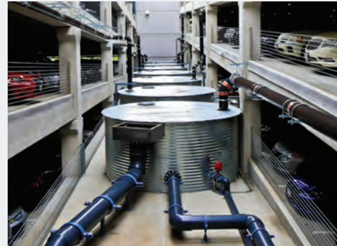
The innovative rainwater harvesting system installed at TMNA’s headquarters campus in Plano, Texas, consists of cisterns in each of the four parking structures. The cisterns, with a total capacity of 400,000 gallons, tie in to a master irrigation system that allows the water to be distributed for landscaping.
